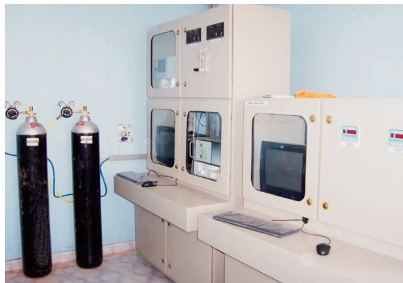
CO 2 supply, recording and monitoring panel
